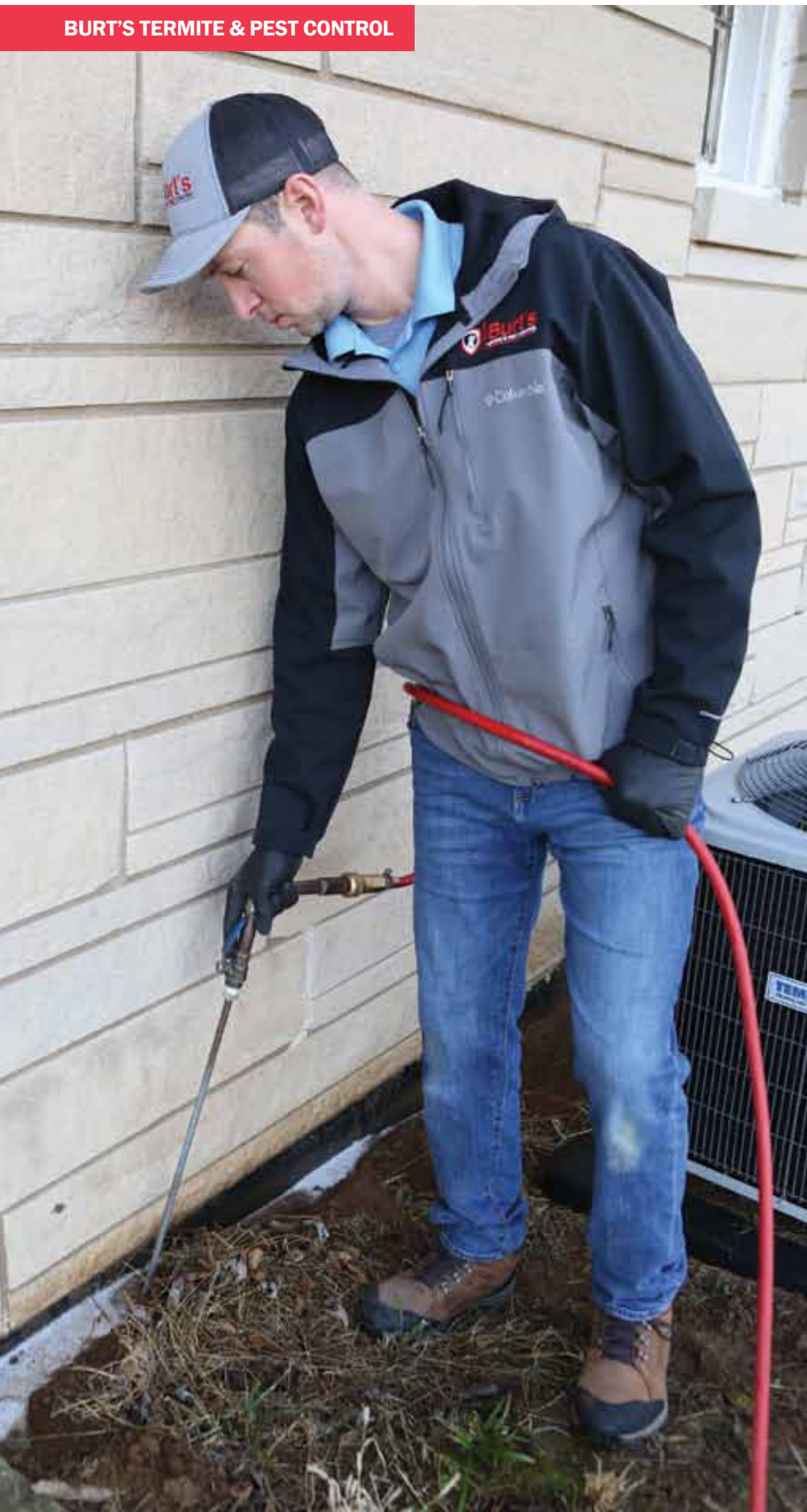
Brandon Foster is shown ground rodding to treat for termites at a job site.
